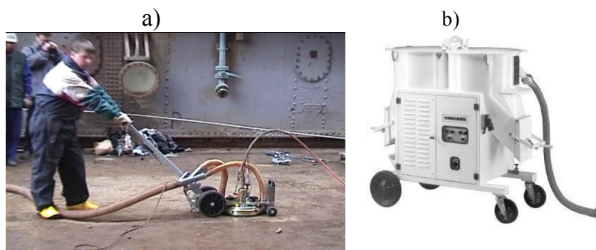
Fig. 14. General view and application of high-pressure trolley AQUABLAST type FRV 3000 (a) and Vacuum Unit type AQUABLAST (b)
