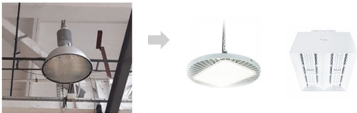
Fig. 9. Transition from the old type of lighting on the left to the modern type of LED lamps on the right
