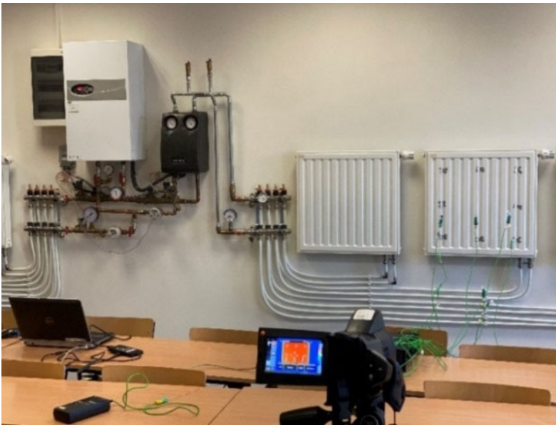
Fig. 1. Lecture room at Kielce University of Technology with tested installation
